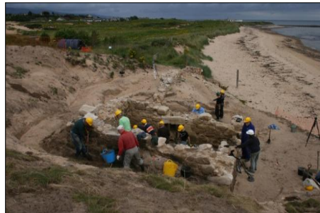
Figure 39: Local volunteers working on the community excavation at the eroding salt pans at Brora, Sutherland. This masonry, buried for hundreds of years in the dune, is the oldest that survives in the village, © SCAPE
